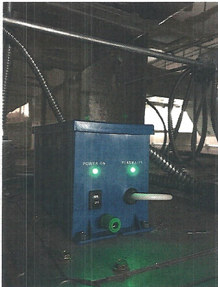
Photograph 1: Bi-Polar Ionization unit installed in the air handler.
